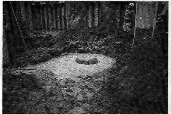
写真-6 湧水状況-2
