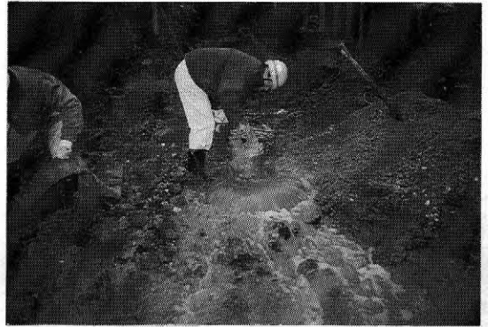
写真-5 湧水状況-1
